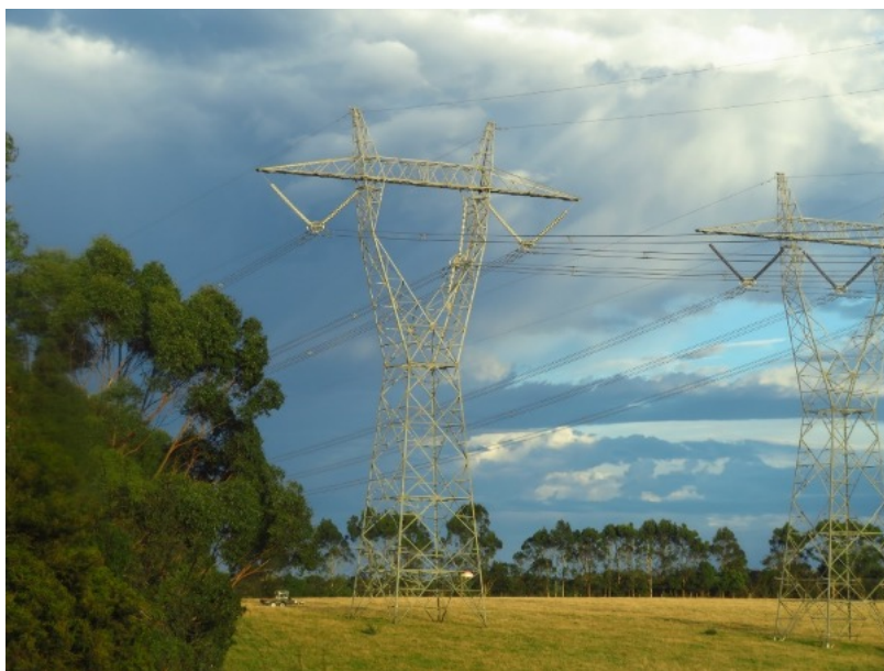
Figure 1: Doulton Insulator Failure T076 HWTS-SMTS #2
