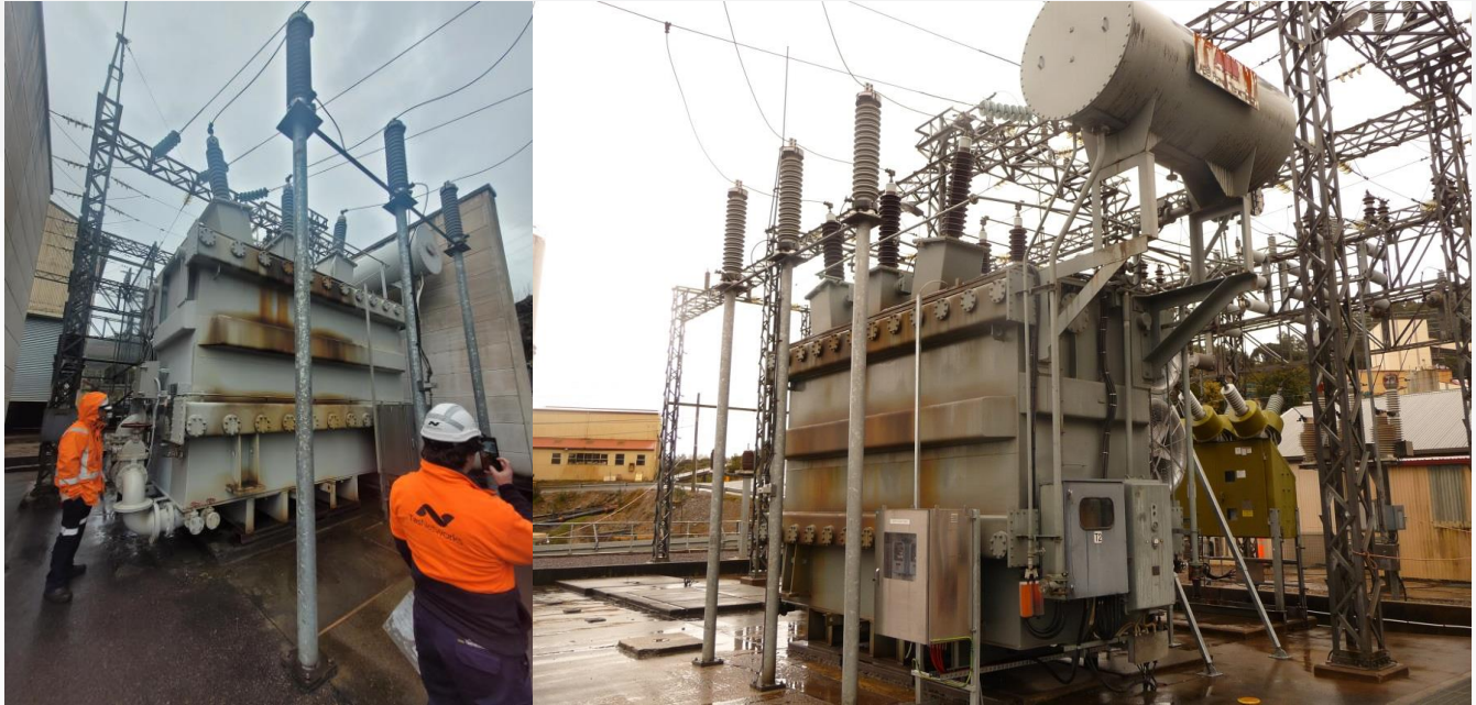
Figure 5: Oil leaks on T1 (left) and T2 (right)
