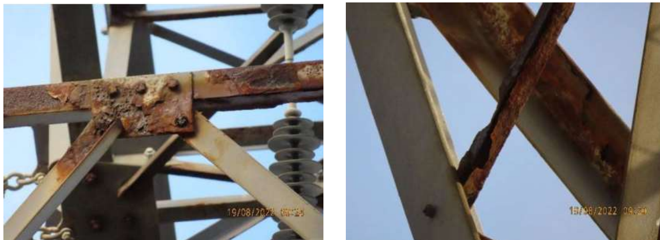
Figure 2: Examples of corroded tower members on the HYTS-APD line
