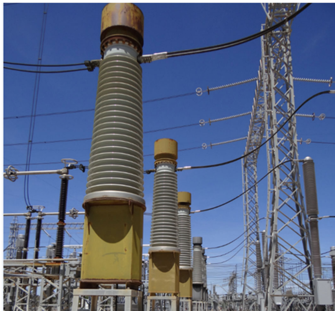
Figure 2 - Endurance 275 kV post current transformers at Torrens Island B circa 1974
