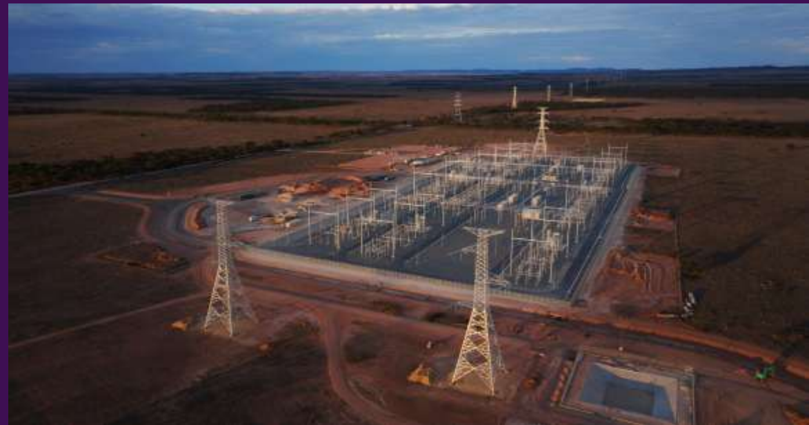
Photo: Bundey 330/275 kV substation
