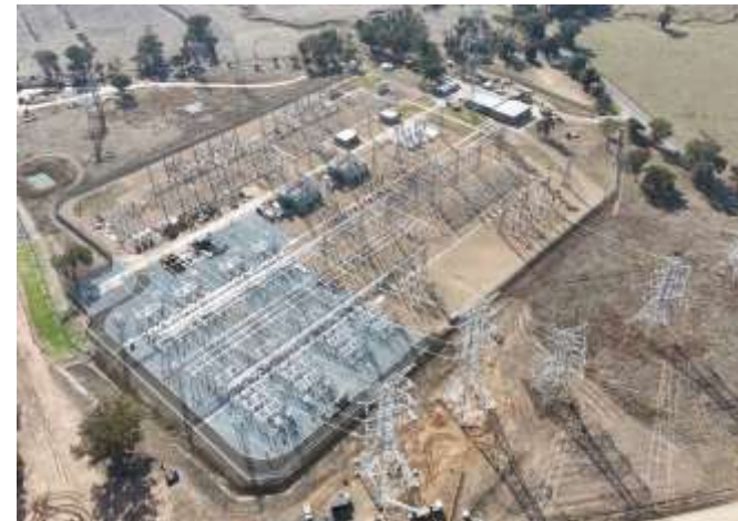
Photo: Wagga 330kV substation
