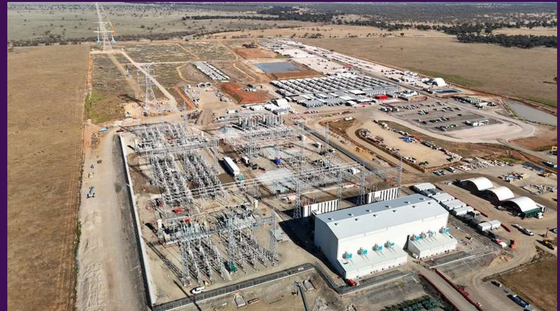
Photo: Dinawan 330kV substation
